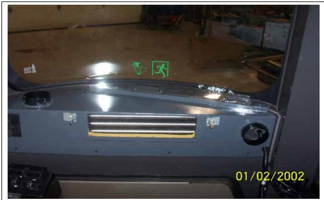
Evaporator cover shown in place. **NOTE: Complete electrical wiring prior to closing the evaporator.**
