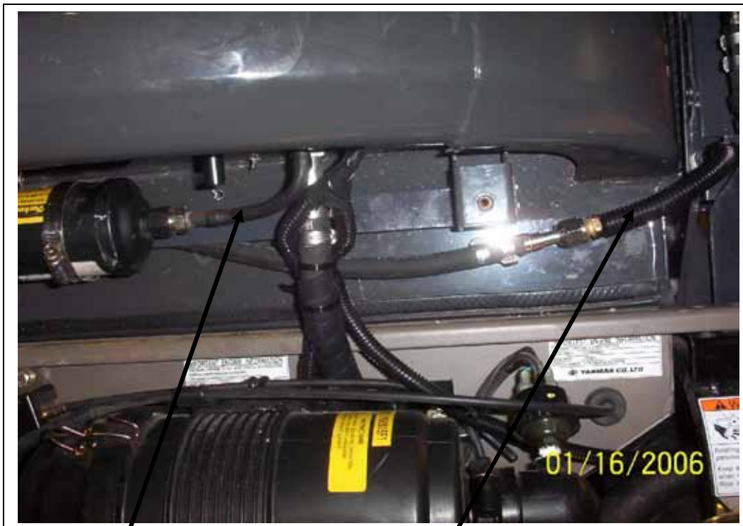
Copper line to expansion valve.
