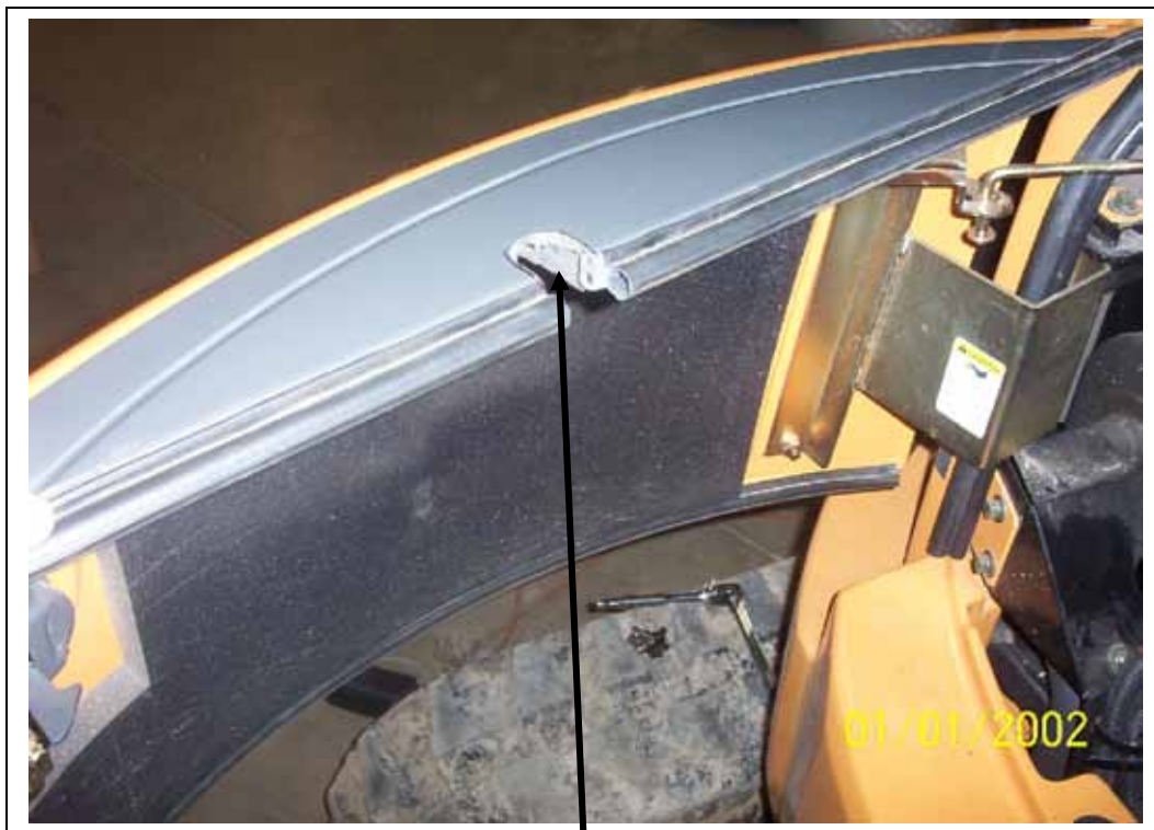
Rear door notched out for hoses and wiring. Install trim to prevent sharp edges from cutting through anything.
